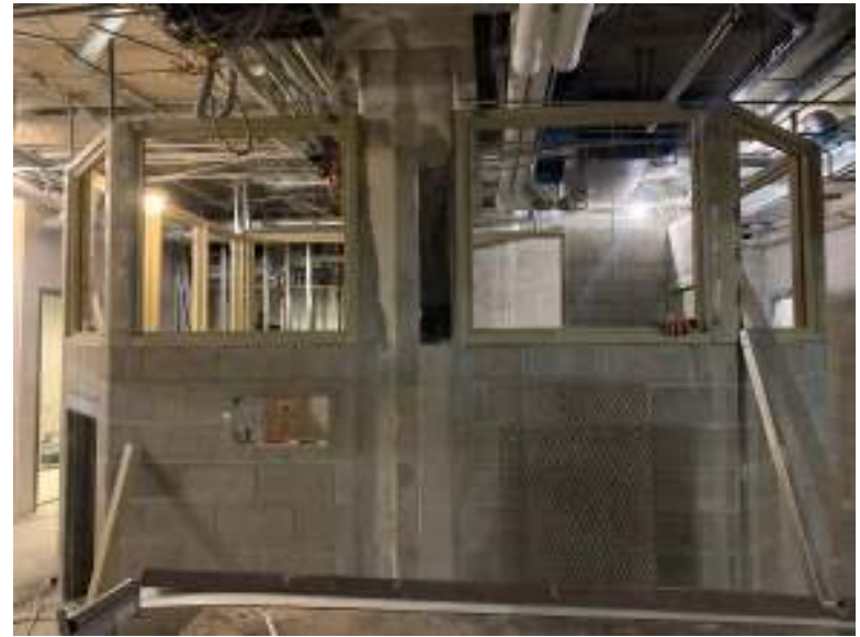
Main Floor – Control Room
