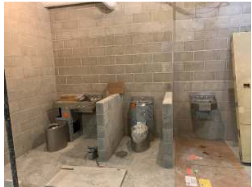
Pod Toilets and Sinks – Pod 1C
