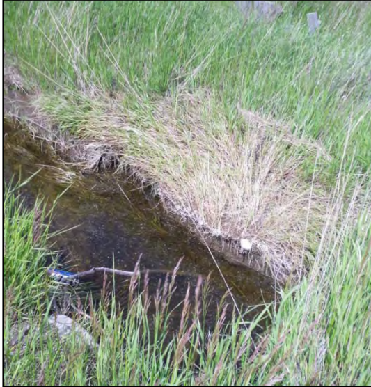
Photo 4.1: Existing cross drain with scour hole located at MP 0.67.
