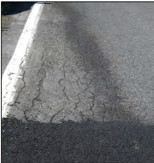
Photo 3.8: Rutting and cracking of asphalt surface.
