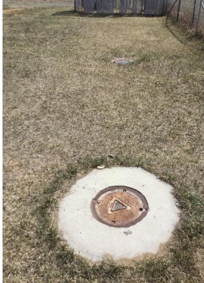
Figure 5: A flush mount well is protected by a steel cover plate that is similar to a sewer manhole cover.
