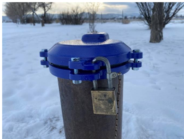
Figure 3: PWS style sealed well cap. The vertical bolts around the perimeter secure
