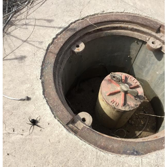
Figure 6: Once the cover plate of a flush mount well is removed the actual PVC well casing and cap are visible. Be cautious of spiders and insects underneath the cover plate.
