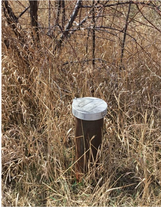
Figure 2: Standard non-sealing well cap on a well.
