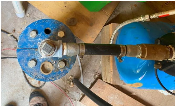
Figure 4: Split well caps are often used with irrigation systems or other permanent plumbing does not require frequent removal of the cap.
